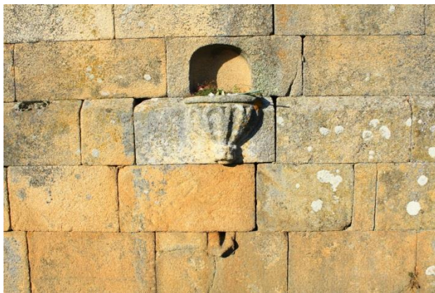
Outdoor of South sacristy where we can see a tank for indoor sink. Original and lovely stonework.
