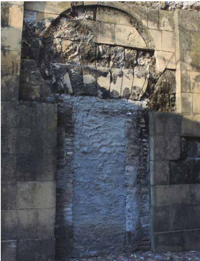
Fig. 9. Córdoba (antigua iglesia de Santa Catalina): acceso al patio de la mezquita, desde la calle, practicado en su fachada suroeste (C. González). / Córdoba (former church of Santa Catalina): entrance to the courtyard of the mosque, from the street, located in the south-west wall (C. González).
