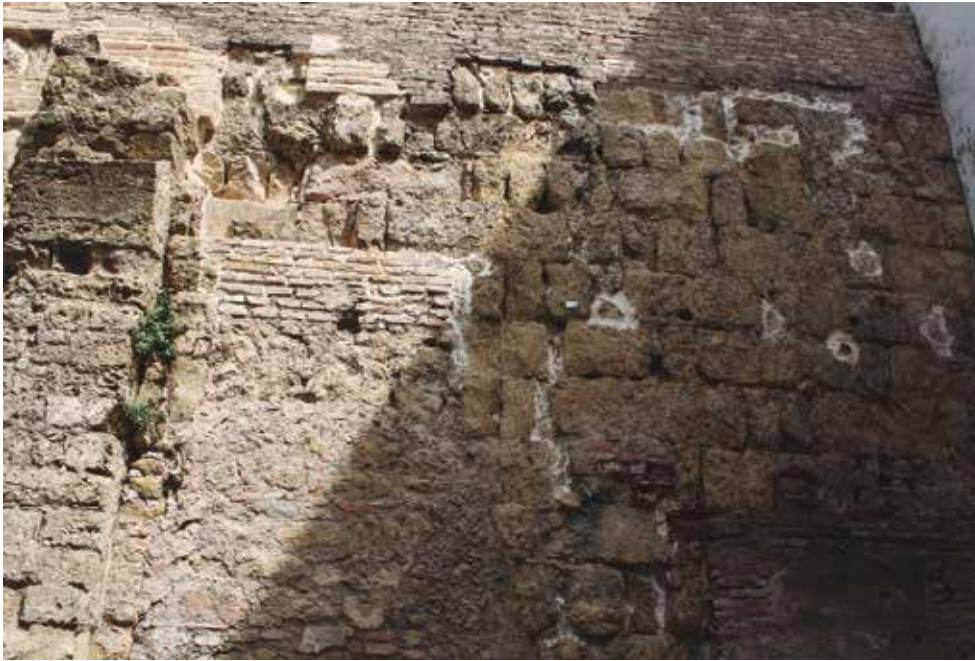
Fig. 8. Córdoba (antigua iglesia de Santa Catalina): vista exterior del muro suroeste, en su tramo correspondiente a la sala de oraciones (C. González). / Córdoba (former church of Santa Catalina): external view of the south-west wall, in its section belonging to the prayer room (C. González).
