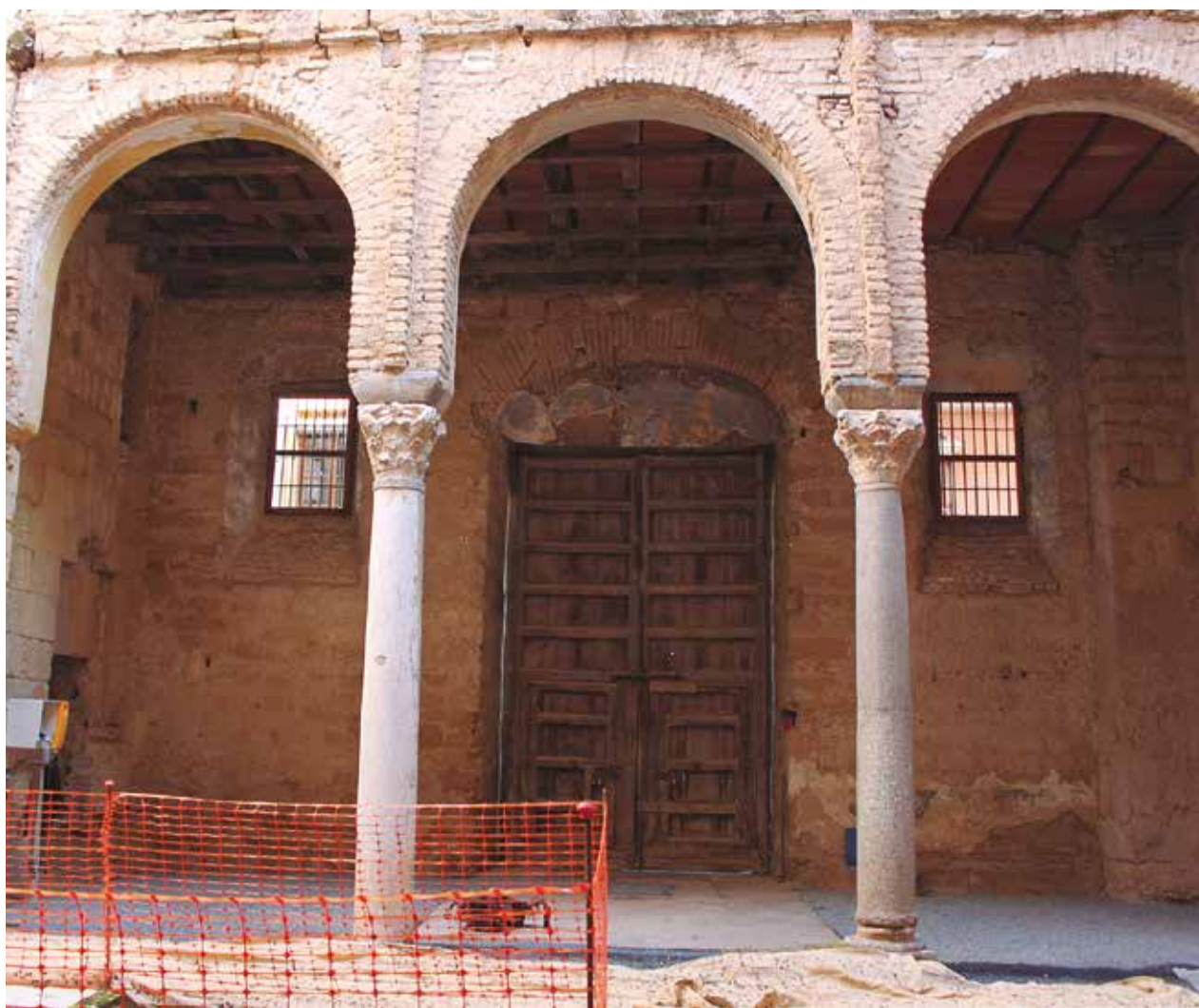
Fig. 10. Córdoba (antigua iglesia de Santa Catalina): interior del patio. La galería porticada que discurre paralela al muro NE de fachada del edificio, y que tiene una simétrica enfrente, ha llevado a pensar en la posibilidad de que el patio de la mezquita contase con galerías en todos sus lados (C. González). / Córdoba (former church of Santa Catalina): interior of the courtyard. The portico arranged parallel to the north-east wall of the building, which has a twin in the opposite side, has led to think that this courtyard could have been provided with porticoes in all its sides (C. González).
